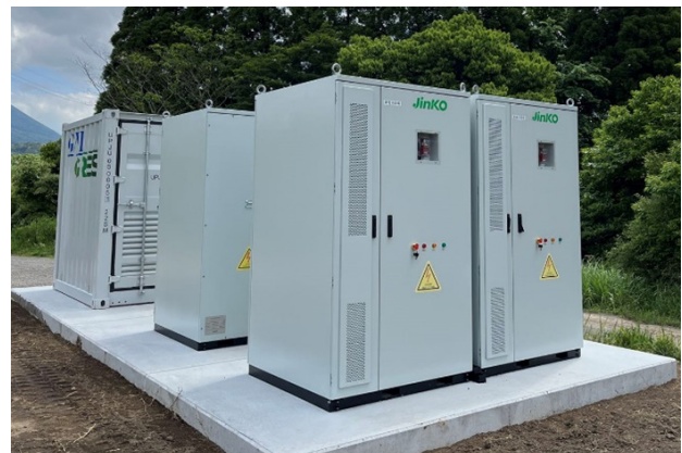
Fig. 2 Jinko ESS 215kWh DC Blocks
